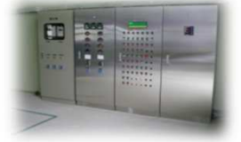
Manual/auto control /commercial power supply
