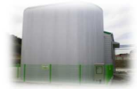
Gas collecting tank
